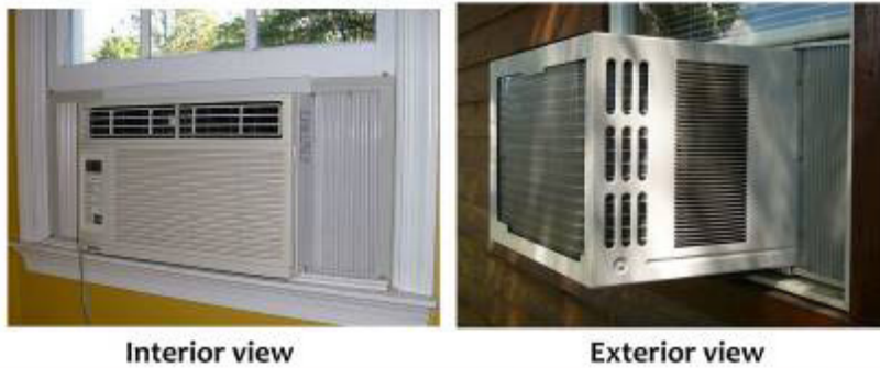
Figure 65 : Interior and Exterior view of Unitary AC
