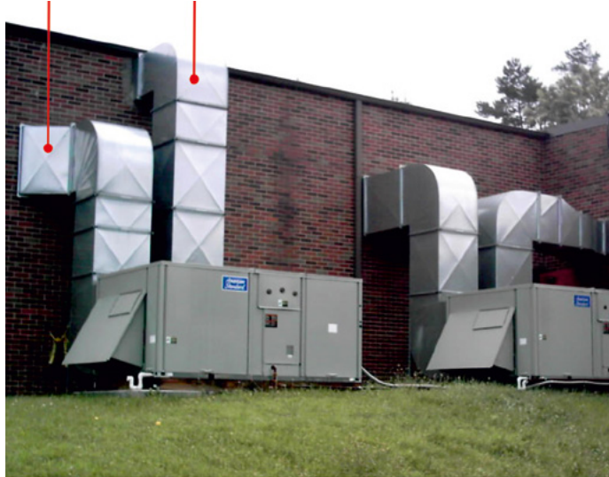
Figure 68 : Packaged air conditioner.
