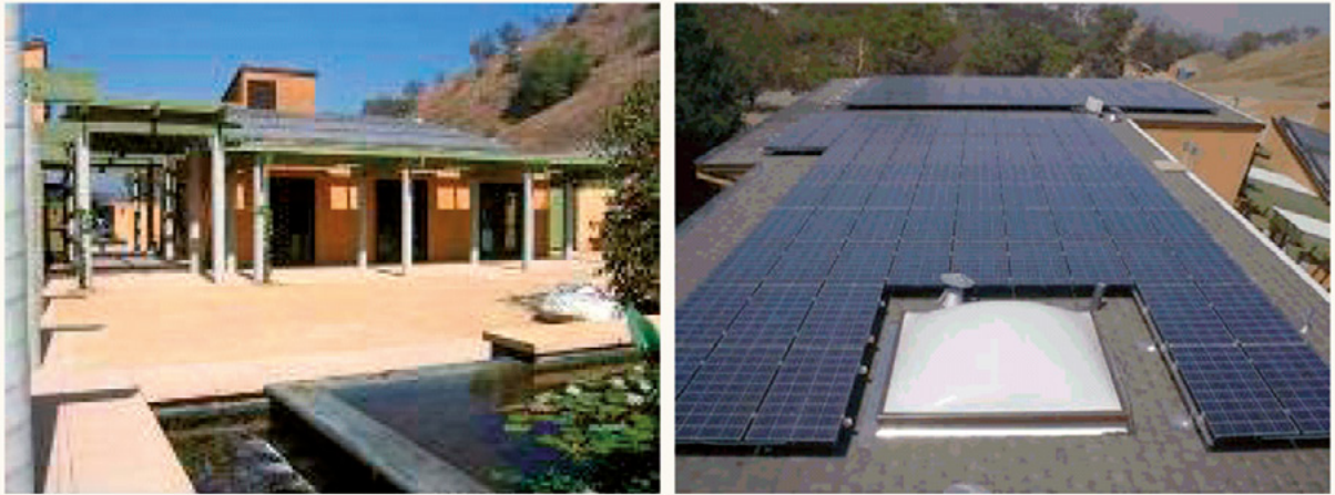
Figure 69 : Solar Power System
